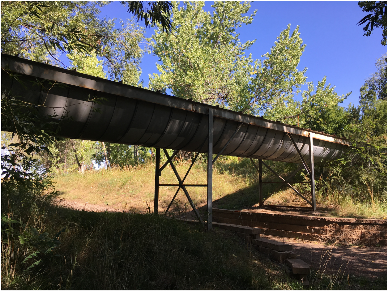
City Ditch Flume over Slaughterhouse Gulch in Slaughterhouse Gulch Park in Littleton. This Flume will never carry Ditch water again.
